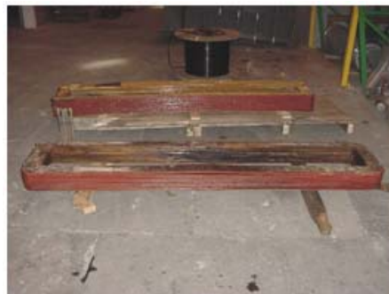
Fig. 1. Overheating effects at the excitation winding. It was burned at rated reactive power excitation.
